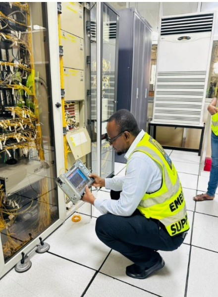
Dr. Godwin at TTCL using ORDR to check fiber link loss
